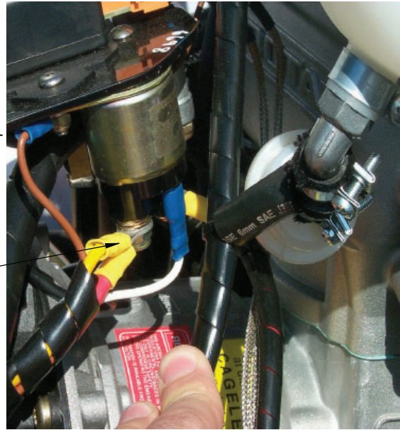
PHOTO SHOWS ATTACHMENT OF WIRES TO THE DATA BOX AND SOLENOID.
